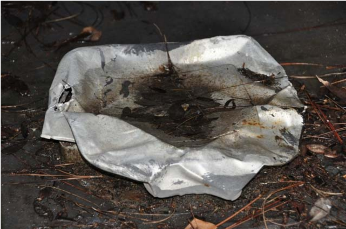
Aluminum ventilation cap under A/C platforms damaged with holes in it. Water penetrating to the space below.
