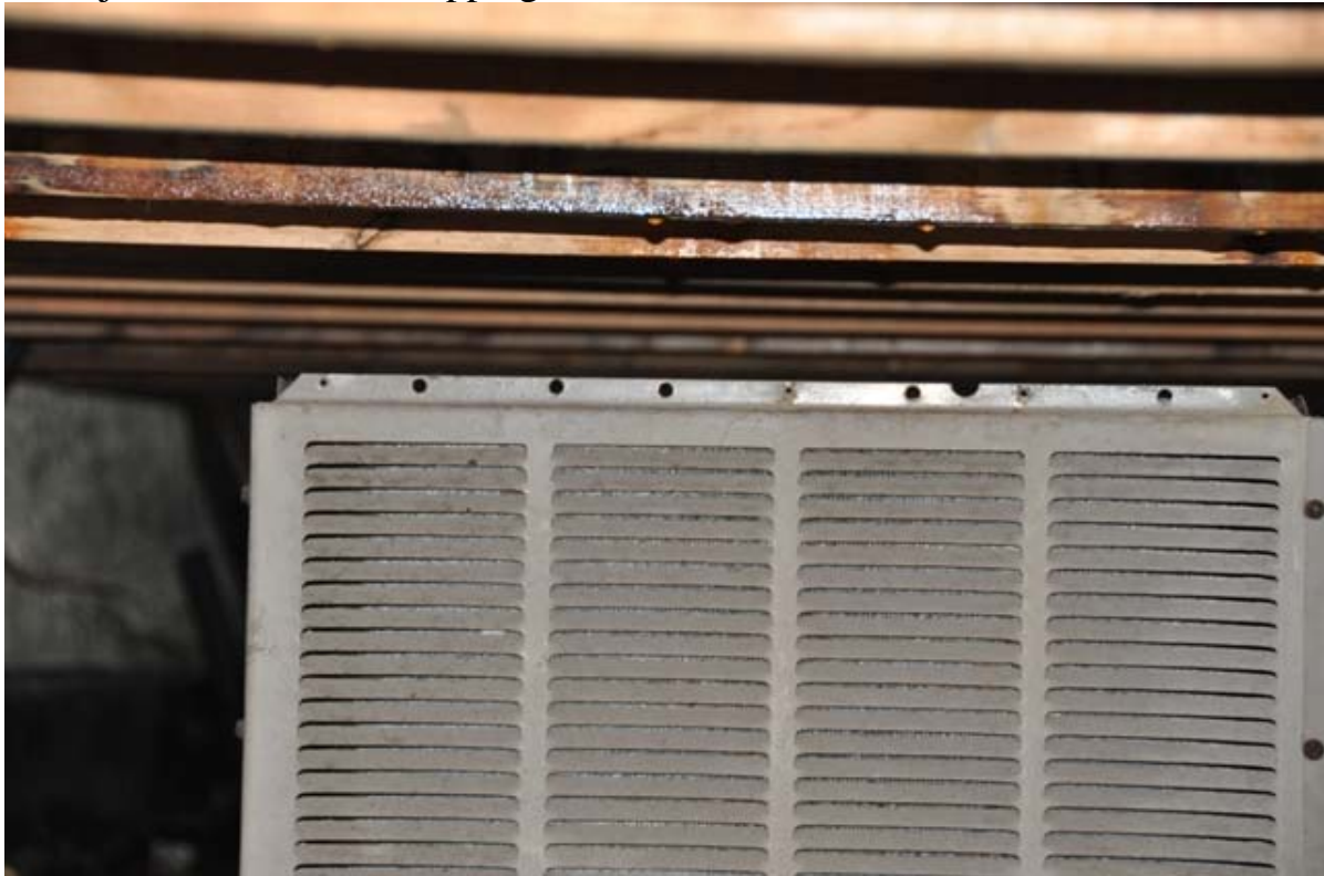
Moisture stains on the roof plywood. Moisture stains on some joists. Bottom parts of some joists are wet and dripping.
